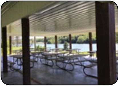
Enclosed metal ceilings and recessed LED lights
